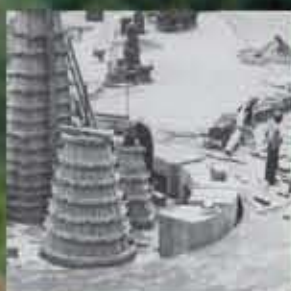
The fountain at Lake Anne Plaza, shown under construction, was designed by James Rossant as an abstract representation of a family and intended to be enjoyed by touching and splashing children.
